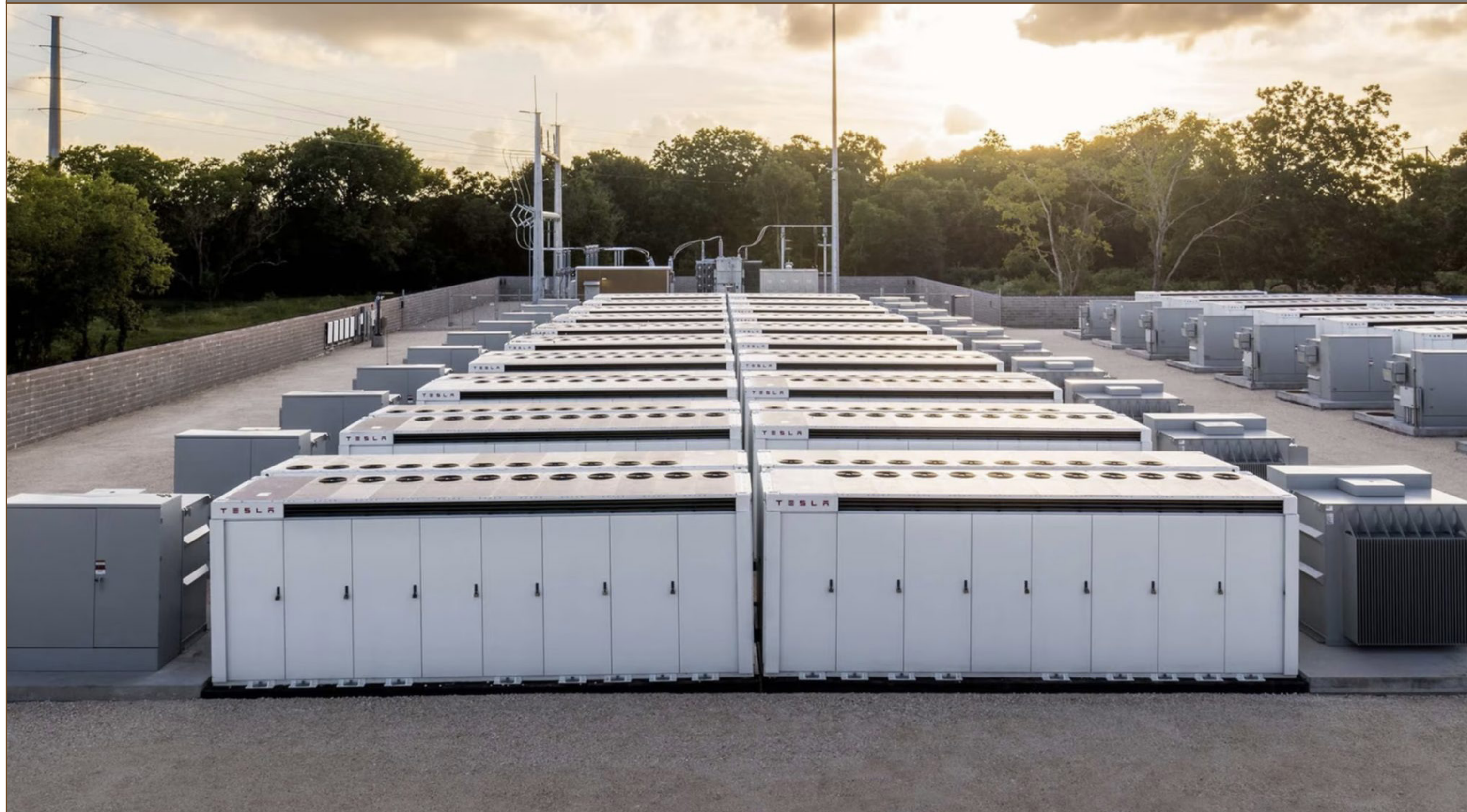
Example of a close-up view of a BESS inside its fenced-in area.
